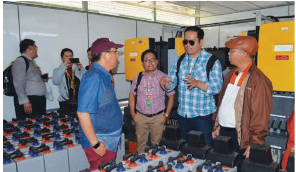
↑ The Honourable Minister inspects the battery and control system for a SARES Solar System.
